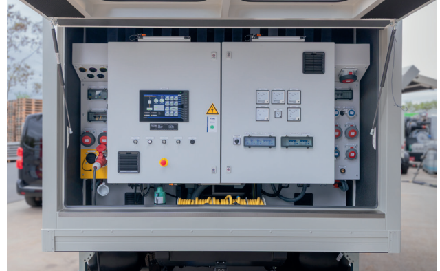
Figure 3: The control centre and the various power connections are located at the rear of the vehicle (Source: Polyma, ifm)
