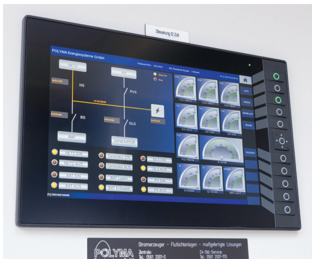
Figure 4: The central ifm CR1204 touch display is used to visualize all operating parameters and to set a wide range of functions (Source: Polyma, ifm)
