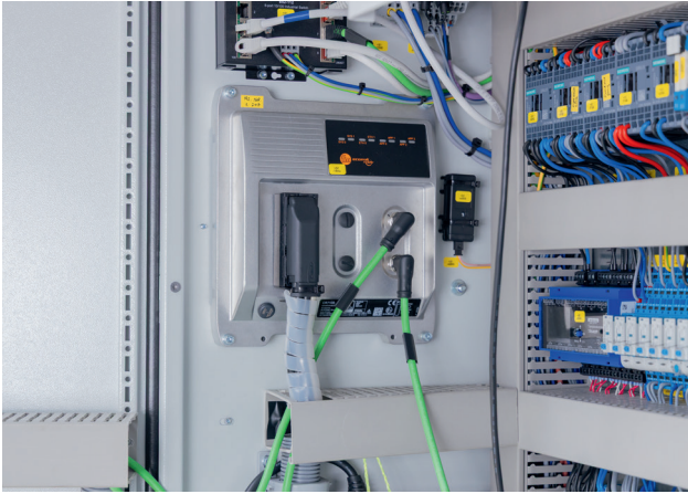
Figure 2: The CR710S central mobile control unit has both a "normal" and a second independently operating safety PLC (Source: Polyma, ifm)
